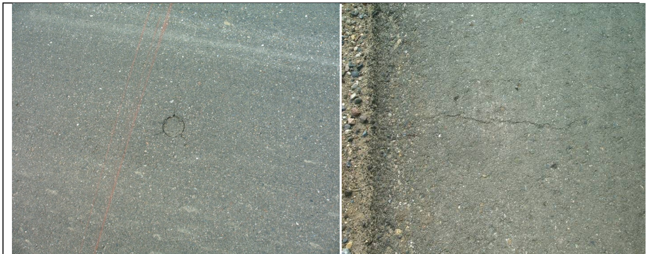
Figure 5.3. Hassan Township: Coring (Left) and Transverse Cracking (Right), March 2008
